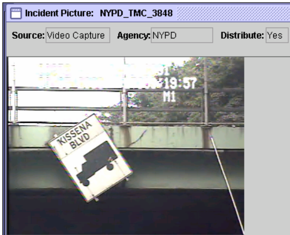
Figure 19. Unsecured Overhanging Sign in Incident 4886.
